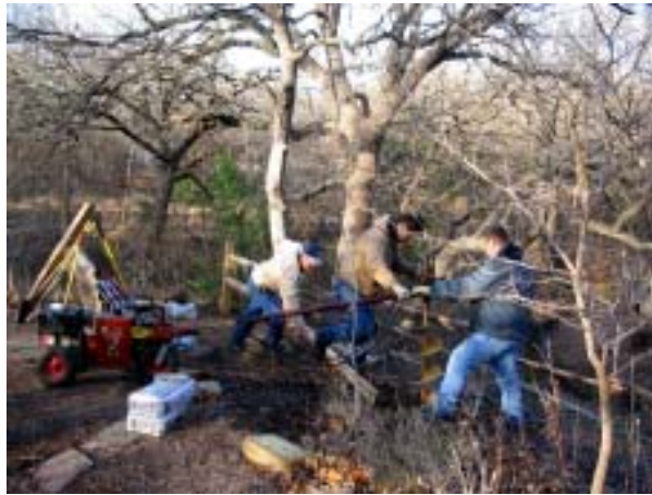
A Parks crew installs a new rustic fence at the overlook bench.
